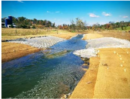
A ford stream crossing was installed to provide a stabilized crossing area.
